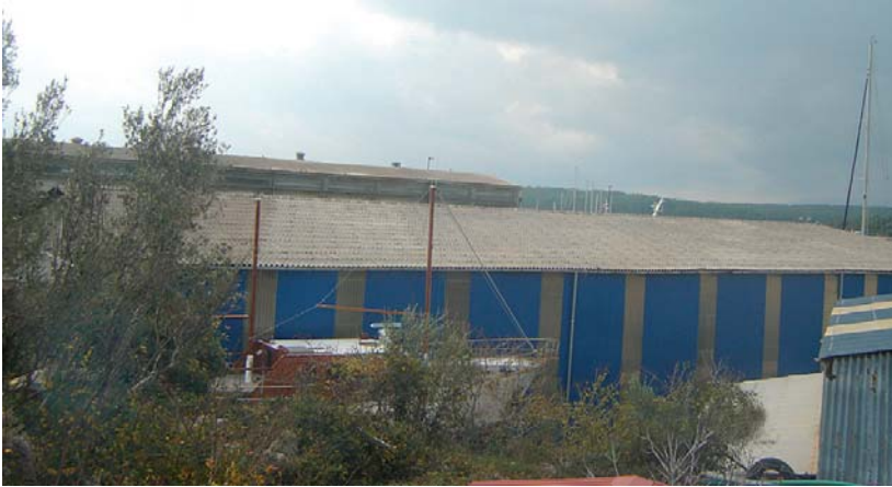
Picture 4 ... and on the roof of the shipyard in Punat on the island of Krk
