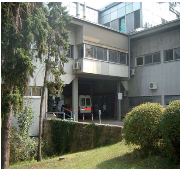
Picture 2 Asbestos panels on the façade of the Clinic for Lung Diseases, Jordanovac, Zagreb
