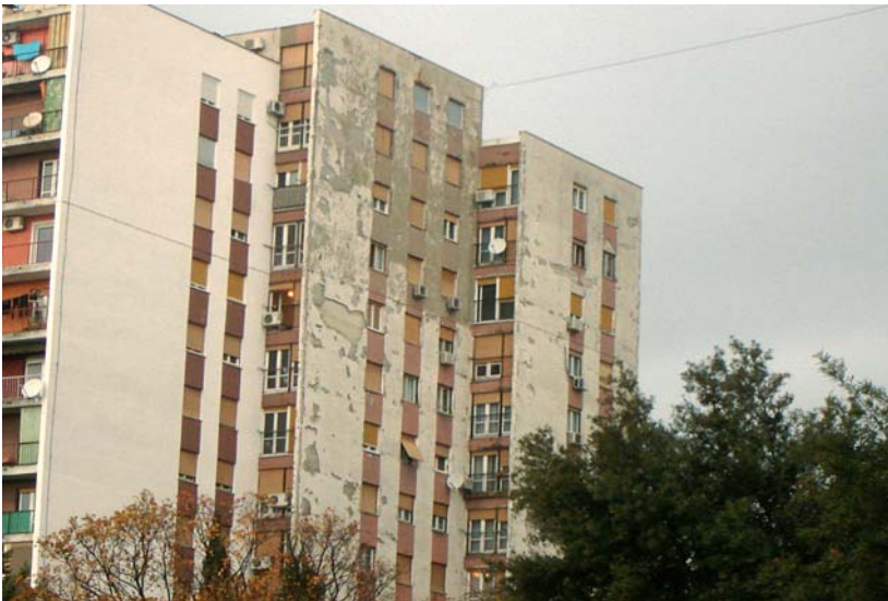
Picture 5 After a number of years of use and with the plaster falling off these high-rise buildings in Rijeka, the asbestos insulation has become exposed
